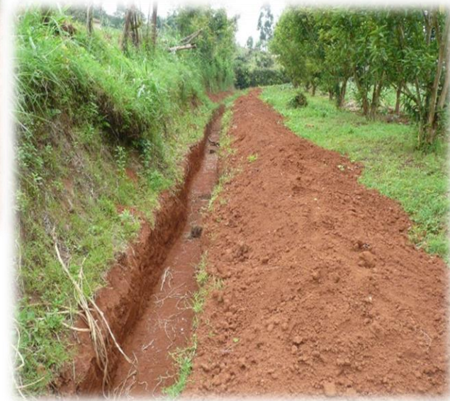
Cutoff drain to protect land from erosion
